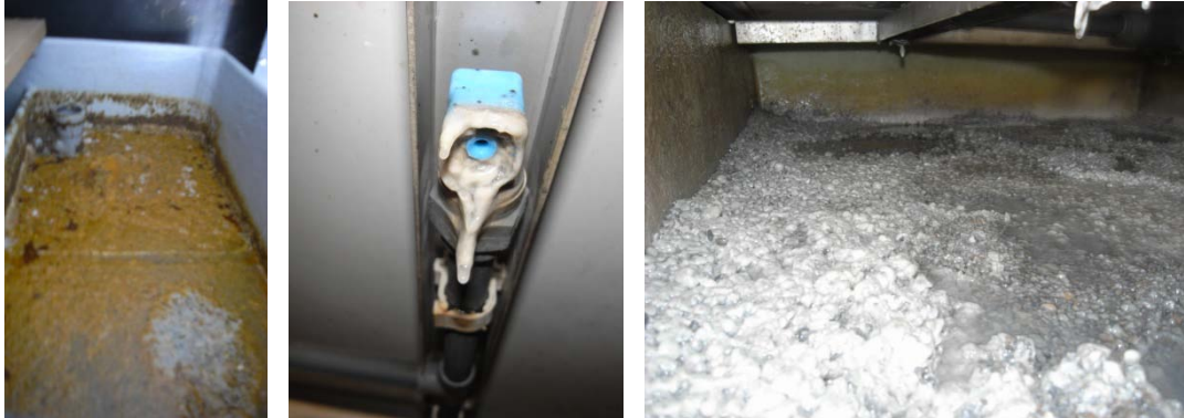
Figure 3: The greywater module was struggling with the high grease content of the kitchen wastewater at Britannia lodge. Despite extremely high loading rates, the system worked for more than 6 months without technical problems and reached a remarkable COD reduction of up to 50%.
