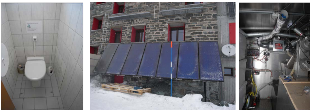
Figure 4: SANBOX blackwater system: A novel combination of Jets VOD TM vacuum sanitation and solar driven SANBOX technology
